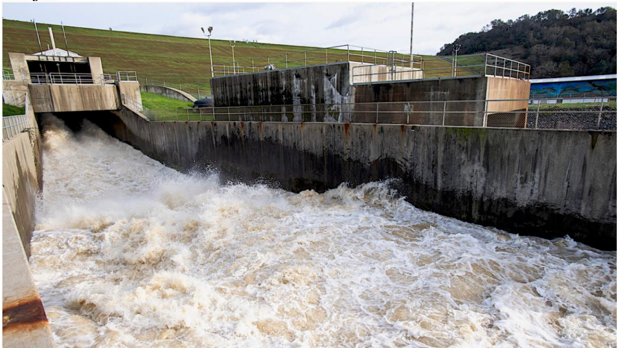
Water being released last month from Lake Mendocino in California following heavy rains. KENNETH JAMES / CALIFORNIA DEPARTMENT OF WATER RESOURCES
